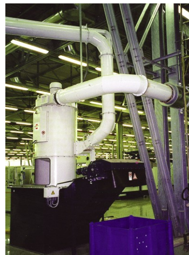
Venturi wet scrubber
