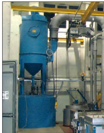
Wet scrubber VDN-T with water holding tank
