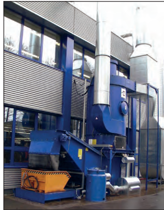
Wet scrubber VDN-AS with de-sludging device
