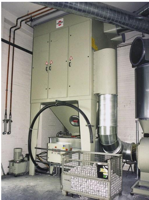
Separation system with dust briquetting
