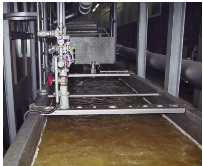
Process water cleaning
