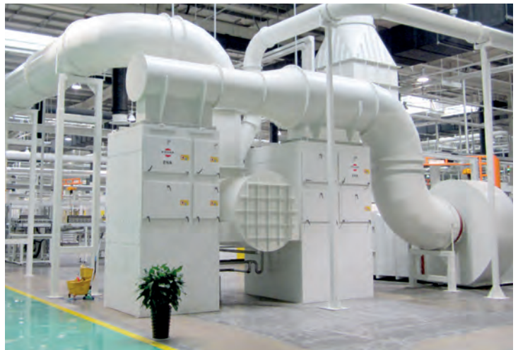
Dust extraction of a truck-engine production with an airflow of 82,000 cfm (140,000 m 3 /h)
