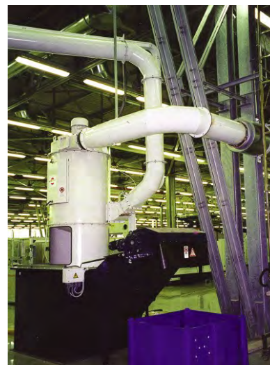
Venturi wet scrubber
