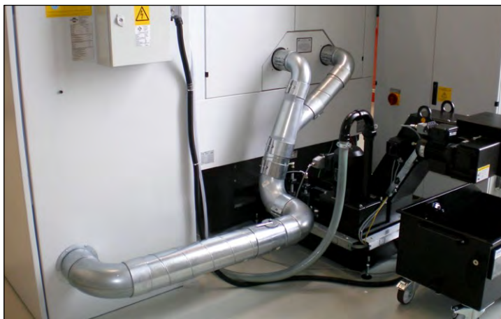
Connection ductwork to machine tool
