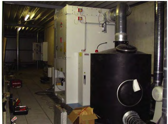
Example of a designed system, L-Cut 4 DOS with activated carbon filter automatic CO 2 extinguishing system
