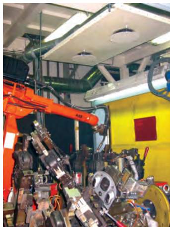
Capturing welding emissions from welding robots in seat component manufacturing
