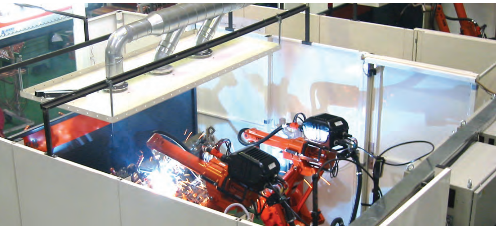
Capturing emissions from welding robots using exhaust fume hoods
