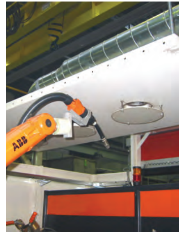
Capturing with exhaust fume hood
