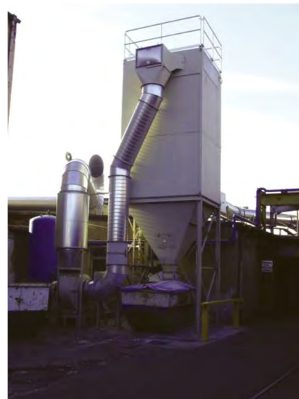
Centralized filter with constructive explosion protection
